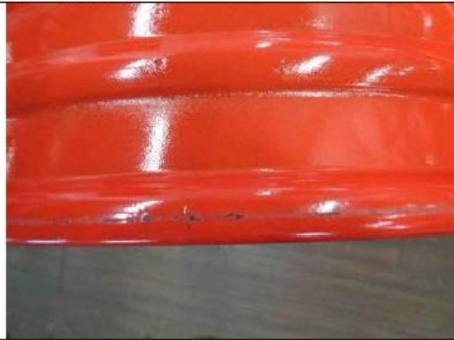
Coating Scuffed off (around 30cm) -Maj
