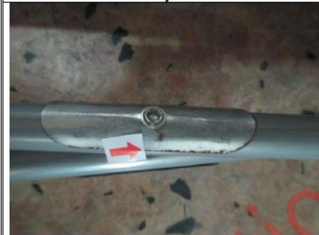
Rust on the pipe Major
