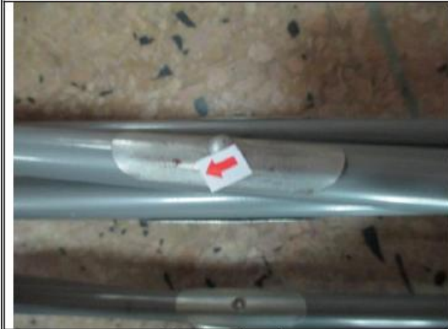
Rust on the pipe Major
