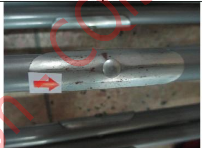
Rust on the pipe Major
