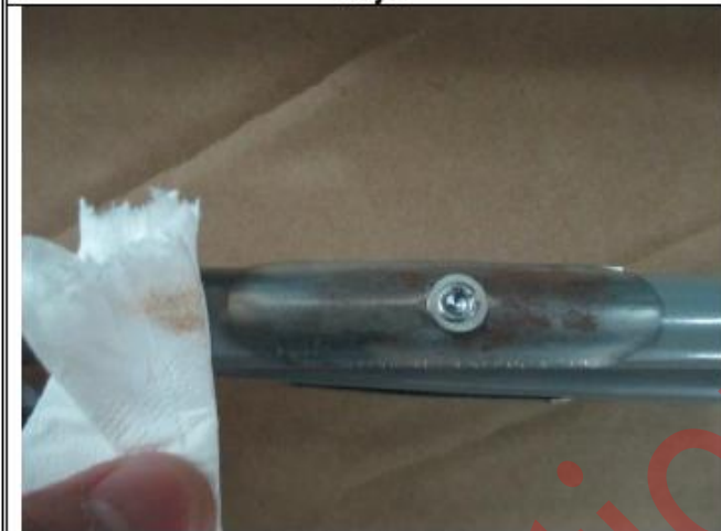
Rust on the pipe Major
