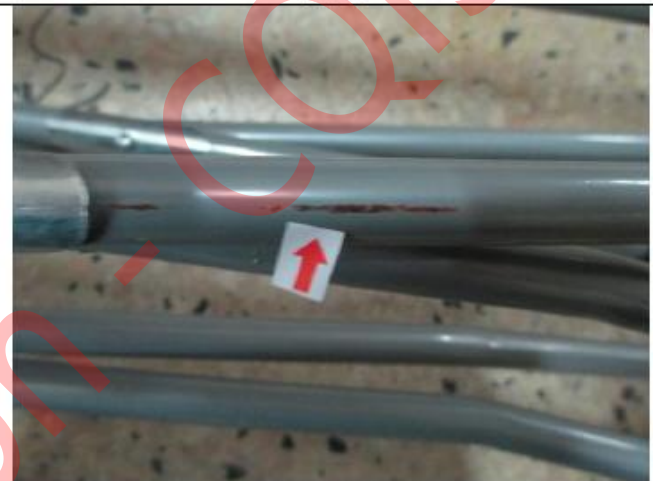
Rust on the pipe Major
