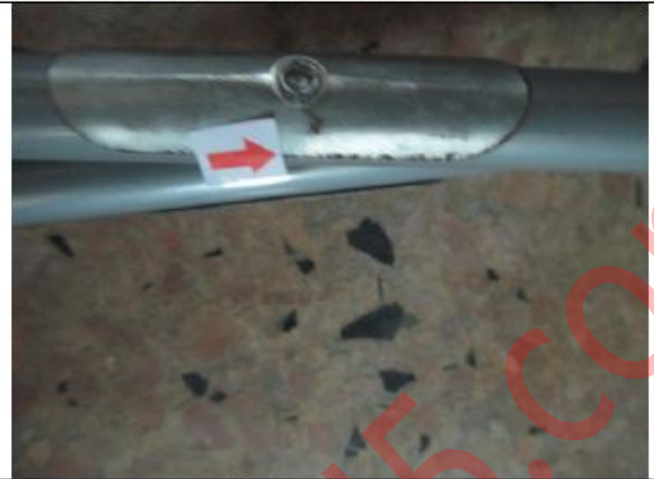
Rust on the pipe Major
