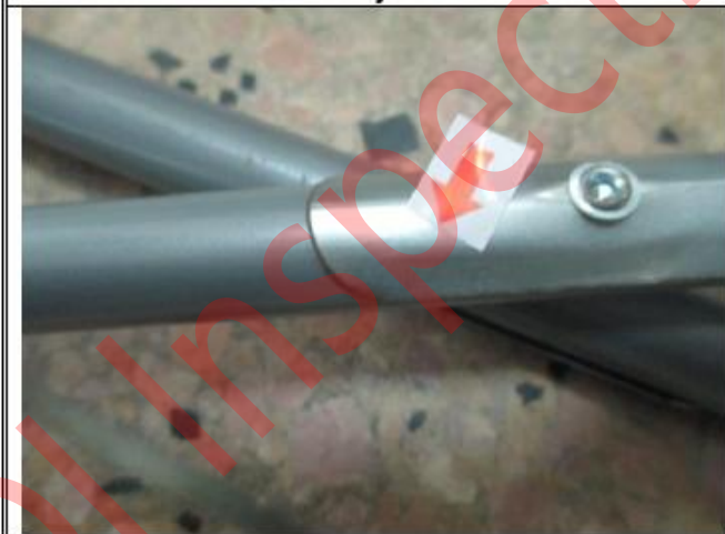
Rust on the pipe Major
